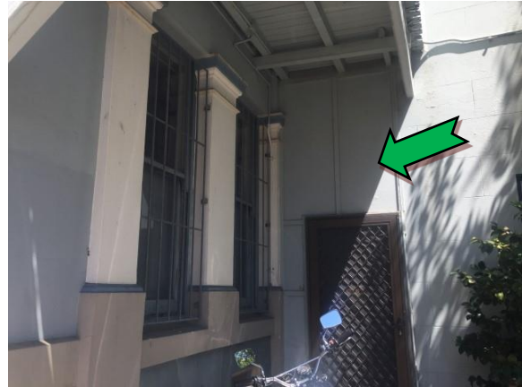
Photo 2. Exterior, ground level, northern entrance, external walls – assumed non asbestos-containing fibre cement sheeting.
