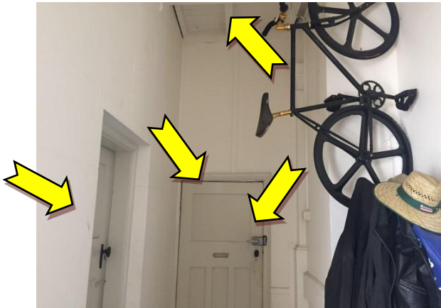
Photo 7. Interior, throughout, walls and features – suspected lead-containing white upper paint systems.
