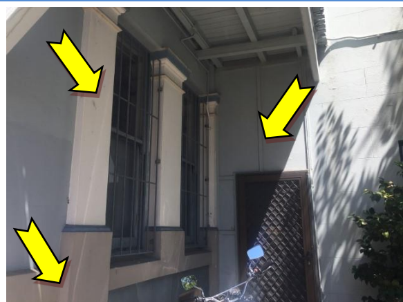
Photo 6. Exterior, throughout, walls and features – suspected lead-containing paint systems (beige, light brown and grey).
