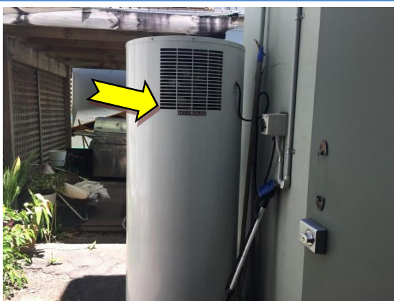
Photo 5. Exterior, ground level, western garden, hot water heater – suspected SMF internal insulation.
