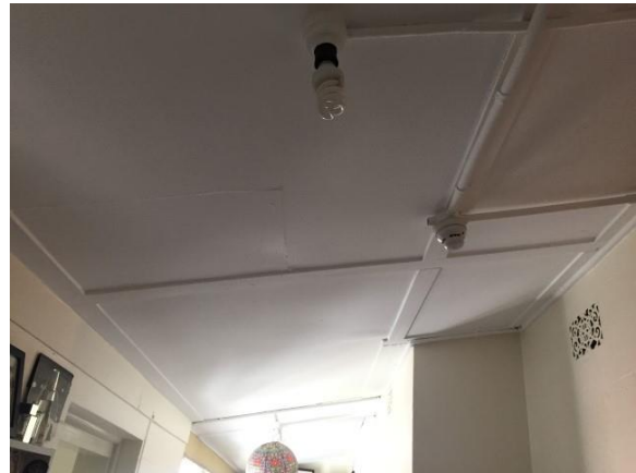
Photo 8. No access – roof space throughout level 1 due to lack of access hatches.
