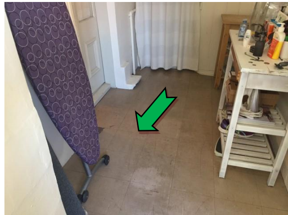
Photo 4. Level 1, western extension, floor covering – non asbestos-containing light brown vinyl floor tiles.
